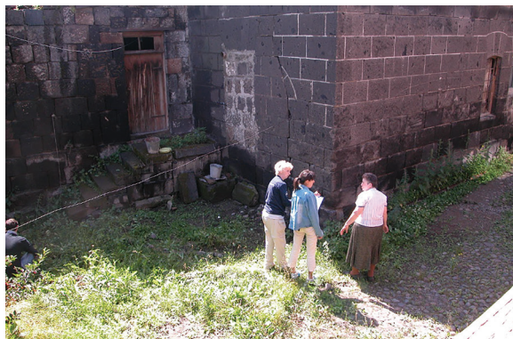
Figure 7.2 Viewing the damage in the rear of the house with the owner and translator
