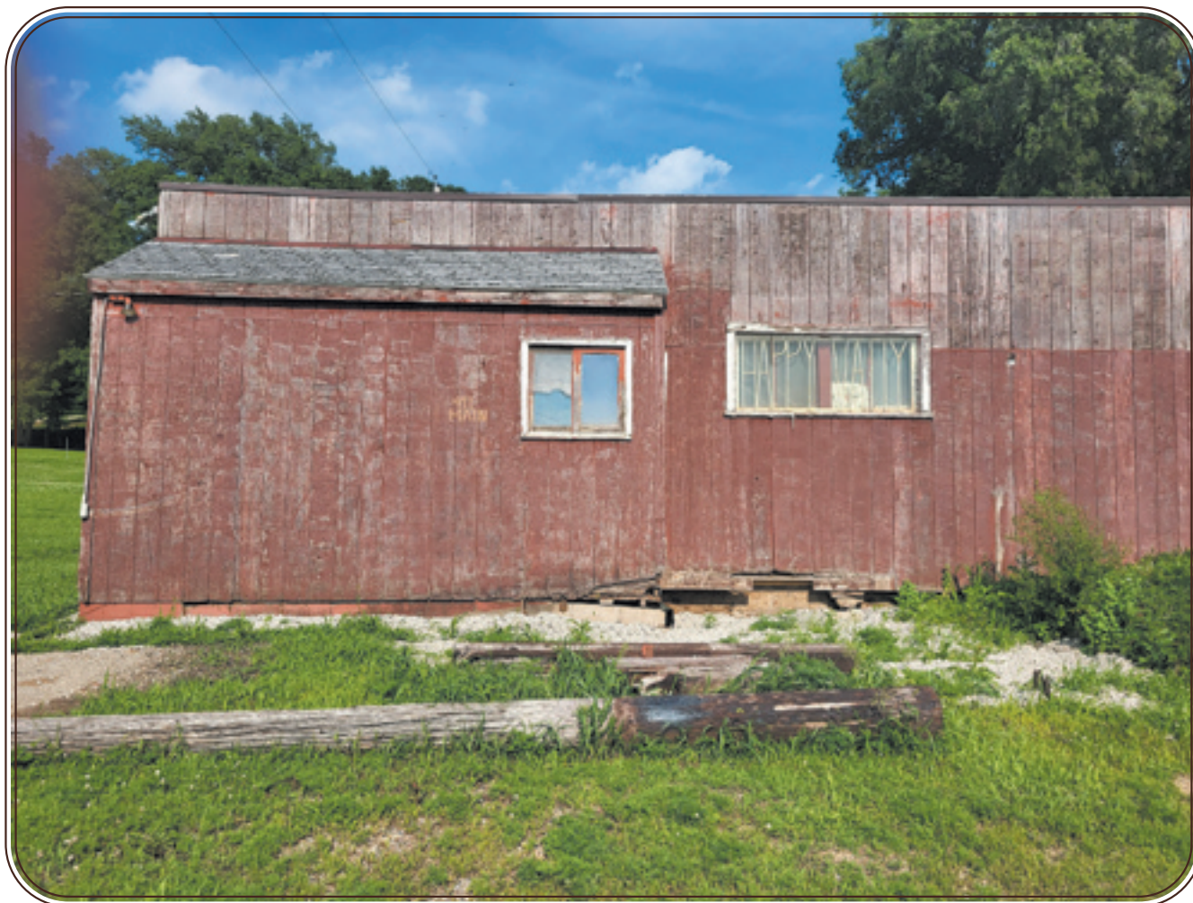
This is the north end of the Rendezvous Bar/Restaurant. The front of the building is dilapidated beyond repair. A sign on the front once advertised: beer, pop, spirits, food, pool tables and a dance floor.
